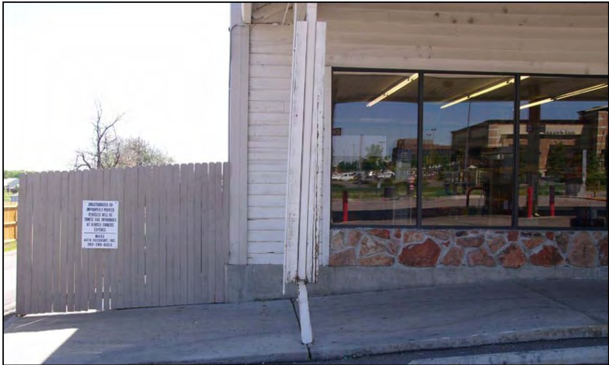
Deteriorated exterior building finishes and support columns were evident in commercial retail properties.
